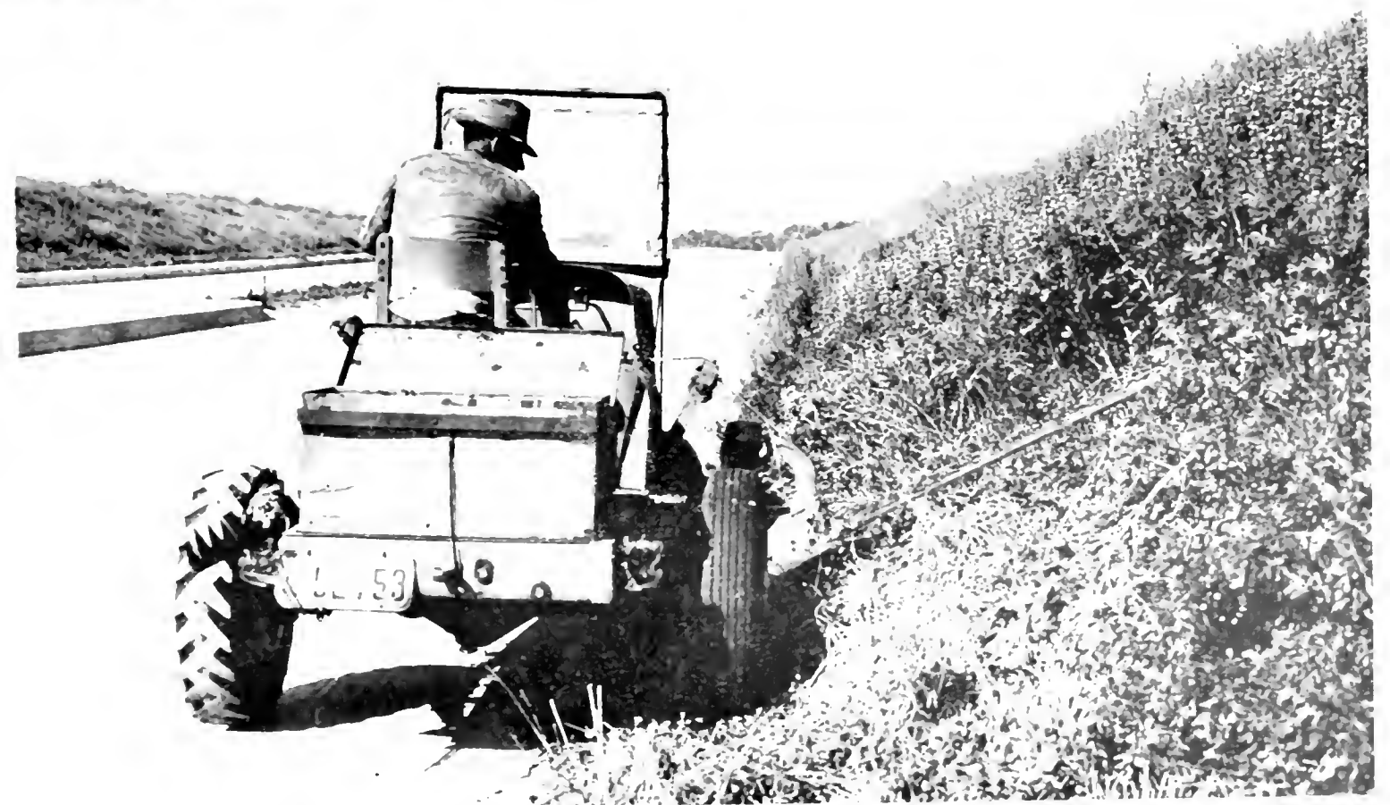
At top—Spraying roadside slope with diesel oil preparatory to burning. Simplified adjustable boom equipment is operated by one man from front of tank truck. Bottom—Mowing tall dry growth reducing fire hazard.
